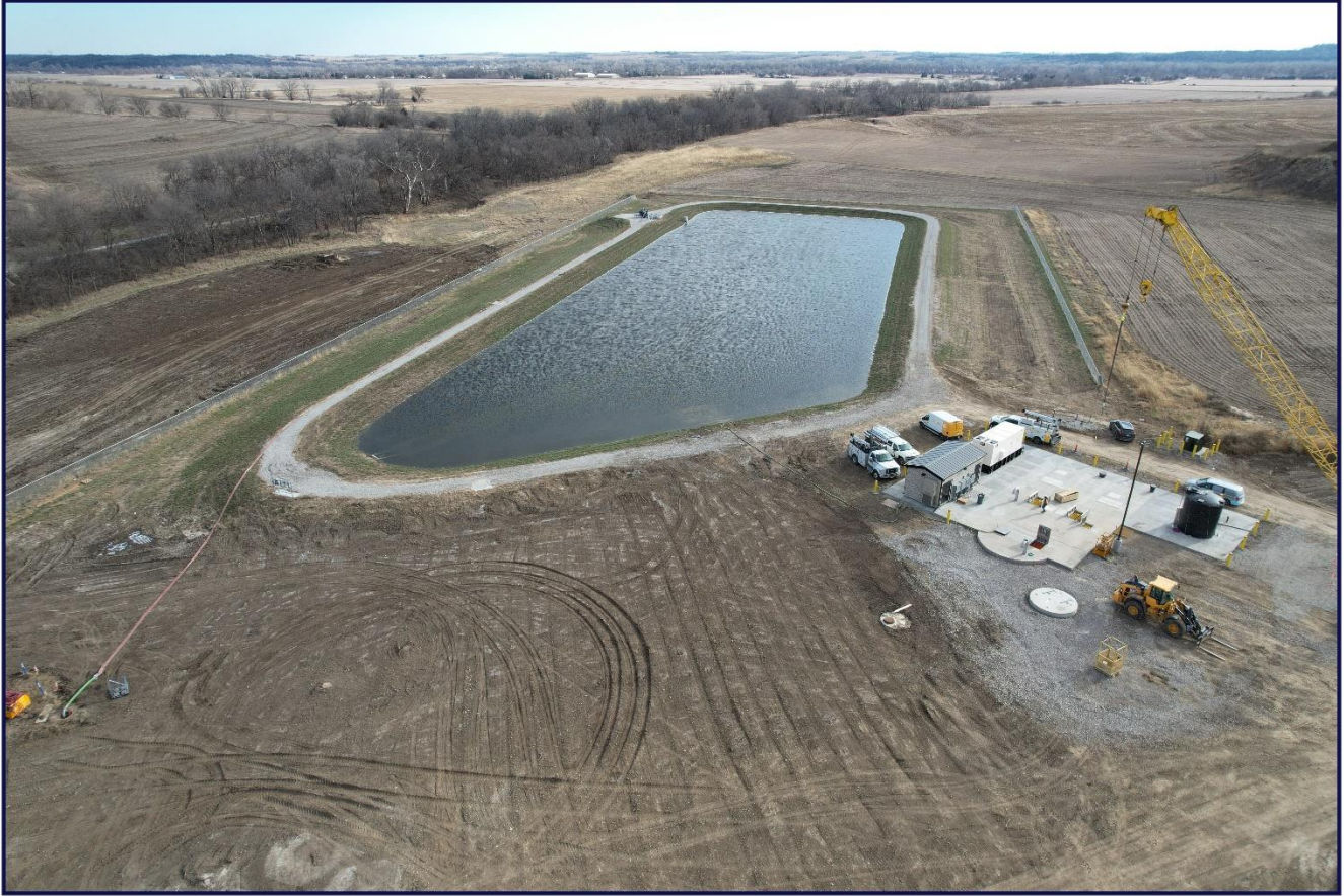
Sarpy County and Cities Wastewater Agency - SCCWWA Phase 1A - Segment 1 and 2 - Lift Station Site Progression - Springfield Creek - Lift Station - December 11, 2024 - Photo 7GPS Position: Lat. 41.064057 Long. -96.135314 Elev. 247.699997 meters ASL
